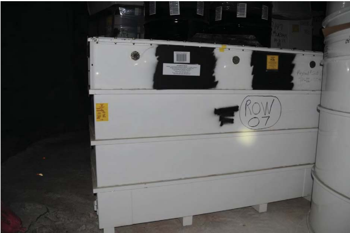
Figure 6 SLB2 in Panel 6 Room 1
